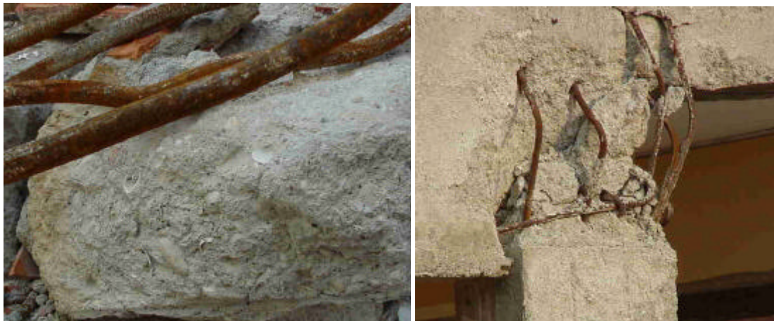
Figure 1 (left) Sea shells in "concrete"
