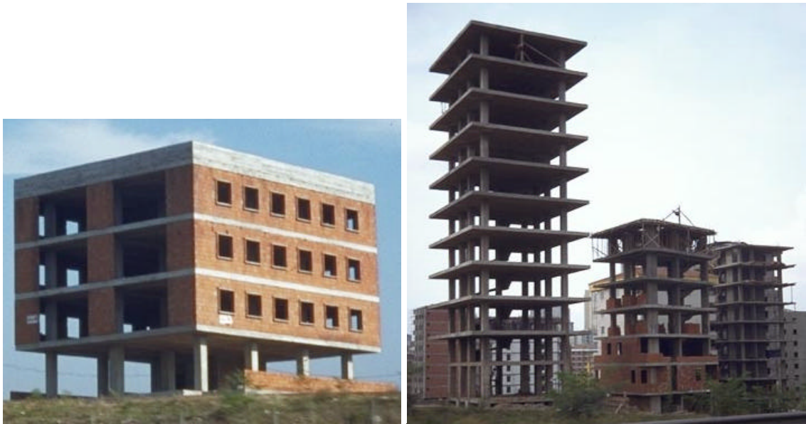
Figures 3 and 4 Buildings under construction alongside the Trans European Motorway between Istanbul and Izmit: cantilevered floor slabs and no shear walls
