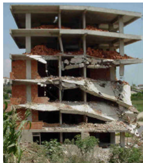
Figure 5 (left) Typical soft storey collapse
