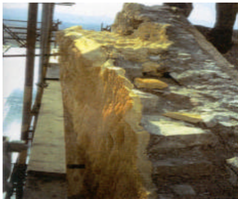
Figure 9: Detail of the damages in the wall of the Basilica
