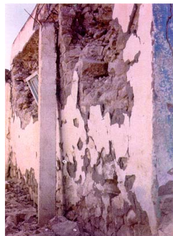
Fig. 8 – Few displacement of the wall in Douar Rwadi.
