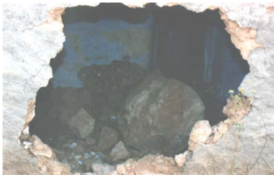
Fig. 5 – Wall destruction caused by rock fall in Douar Tafensa..
