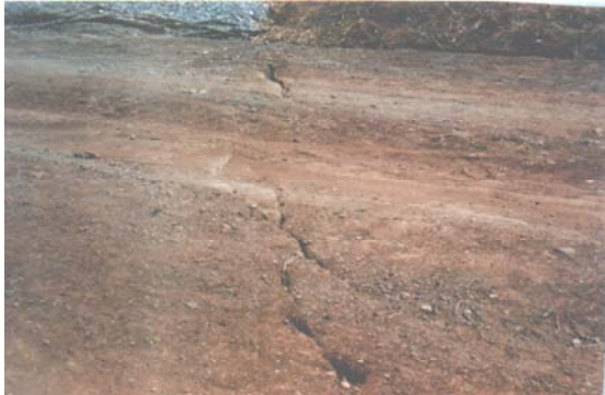
Fig. 3 – Fissures affecting ground in Tanda Ifran.
