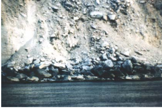
Fig. 2a- Soil falls in the coast cliffs of the Mediterranean Sea west of Al-Hoceima city.
