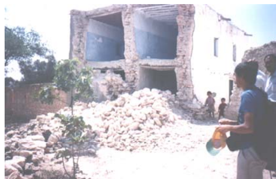
Fig. 6 – Adobe construction strongly affected by earthquake in Douar Tafensa.
