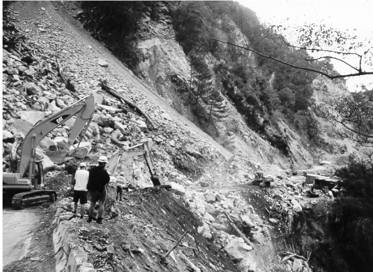
Figure 7. Clearance of rock slide debris from I8 near Techi
