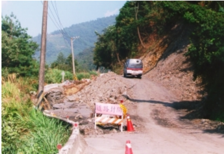
Figure 3. Damage to highway 8 by a seismically-triggered landslide near Lishan
